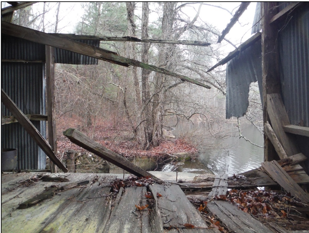
Figure 15. View of south spillway at top of dam at the McCallum Mill (MG0153) property, from mill building, facing north.
