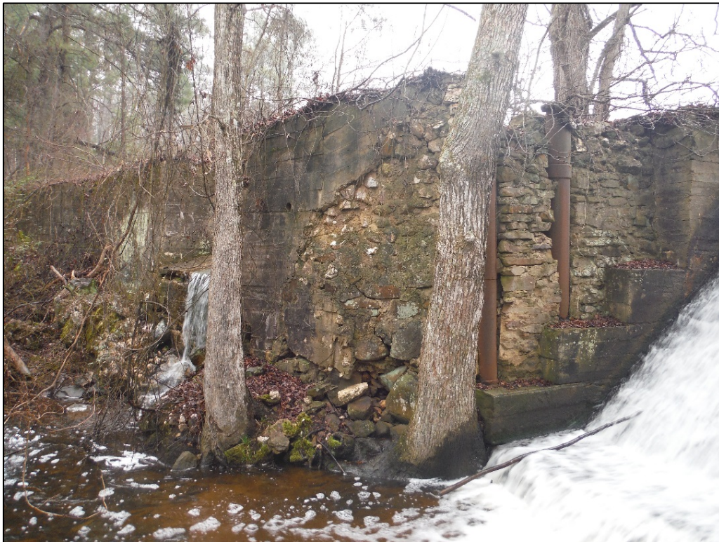
Figure 13. View of central portion of dam at the McCallum Mill (MG0153) property, facing northeast; south spillway is in the foreground (right) and north spillway is in the background (left); metal piping is built into the stone dam on the north wall of the south spillway.
