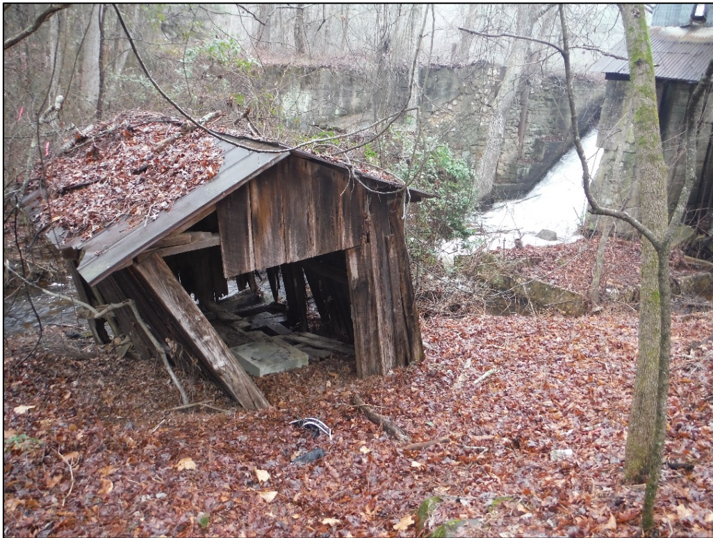
Figure 12. View of building ruins and concrete foundation at the McCallum Mill (MG0153) property, facing northeast.
