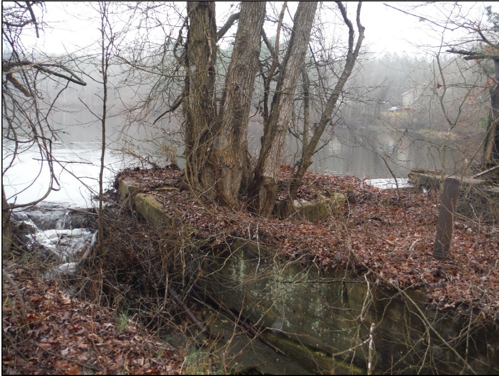
Figure 14. Central portion of top of dam at the McCallum Mill (MG0153), facing east; north spillway is in the foreground (left) and south spillway is in the background (right); a metal pipe extends out of the central portion of the dam and cut stones are beneath the leaves.
